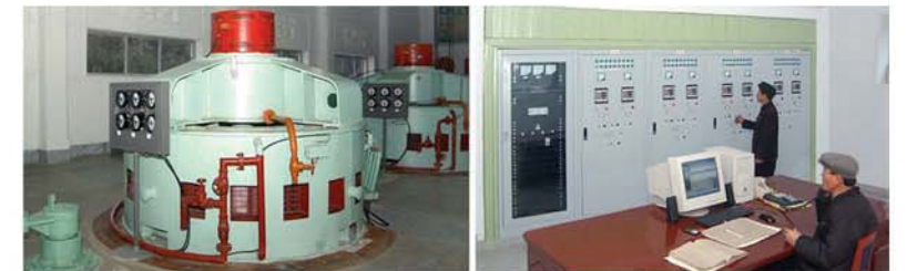
Minor hydroelectric power plants are set up to contribute to power generation.
