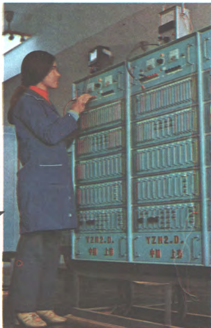
The control center of the power stations
